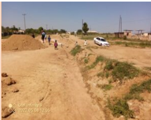
The contractor heaped gravel on the road before abandoning the project for over six months now making it difficult for motorists and residents to rush their patients to Musiso Mission Hospital.
