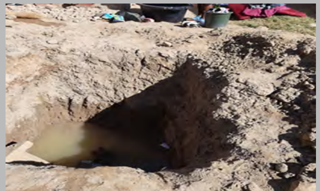
Figure 15: One of the open pits left by Mutare City Council in a bid to repair burst water pipes
