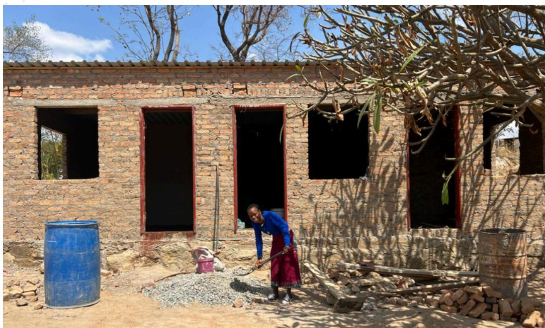
Picture of the week: Grace Chivere is building her own house through the Sustainable and Resilient Rural Livelihoods for Women and Girls program
